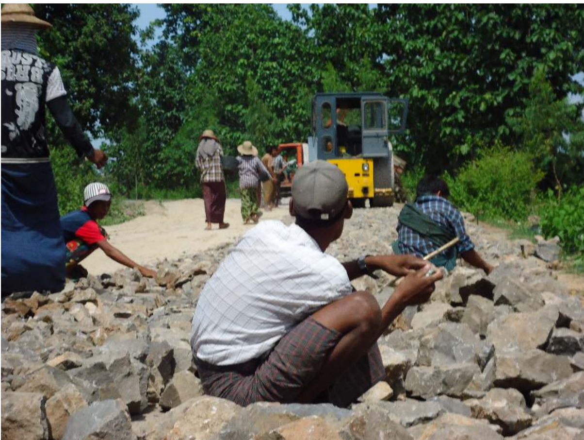
A road under construction near Alauktaw Kathapha National Park, near Kani, Monywa. This particular road was built through a formerly protected area and will link India's Infar City and China's Kunming.
